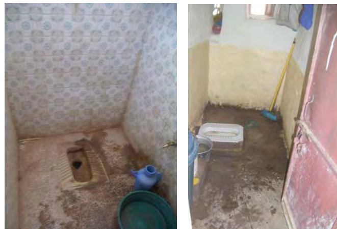
Figure 10: Toilet rooms with water cans for flushing
